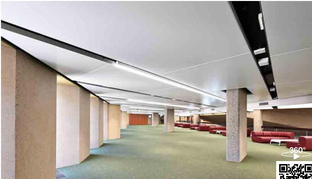
≈ 400 m 2 Barrisol Radiant Cloud Clim®
