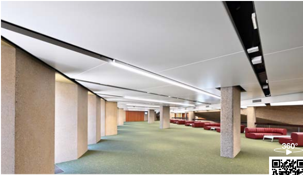
≈ 400 m 2 Barrisol Radiant Cloud Clim®
